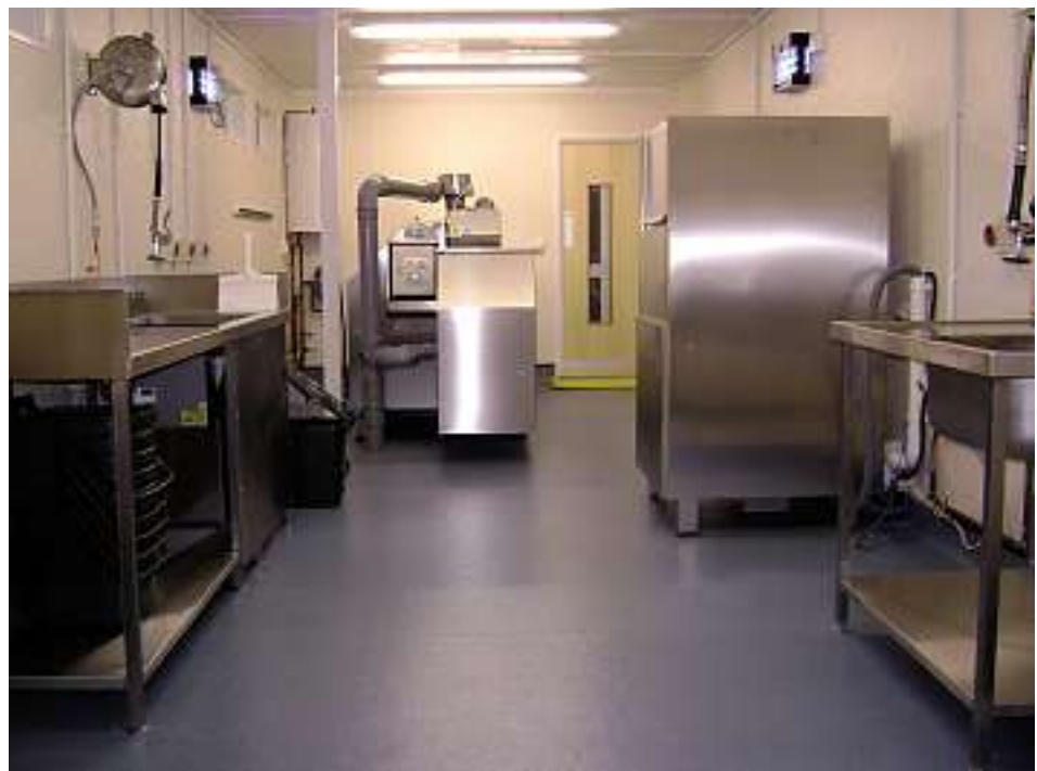
Food waste is first emptied from the waste collection bins on to the sorting table before being pushed into the hopper of the FWD. The captured dewatered waste is then loaded into the IVC. A utensil washer ensures the bins are kept clean.
