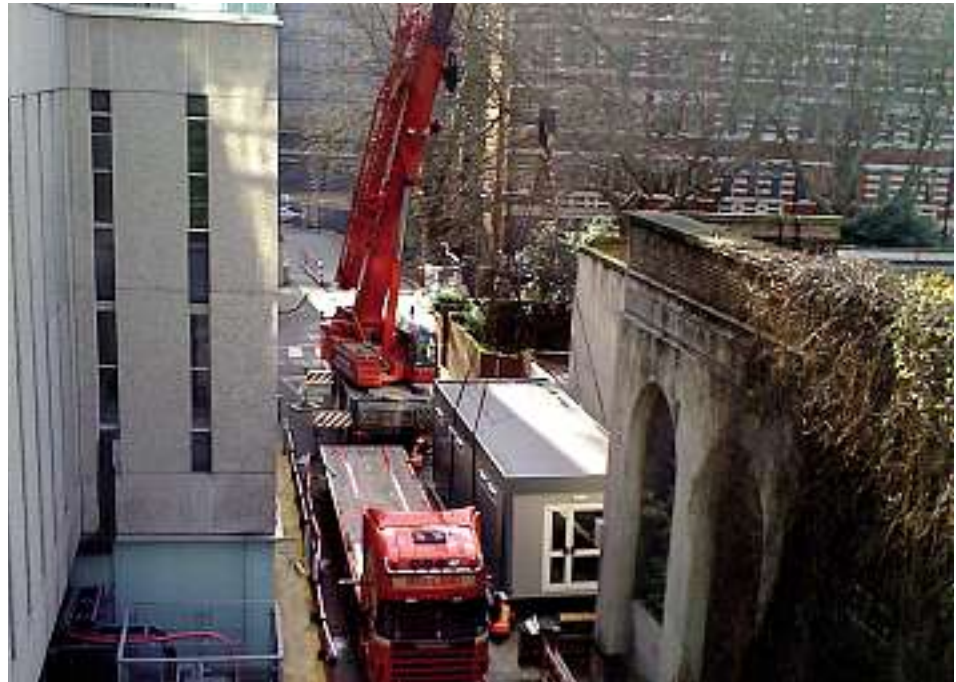
The CompPod is delivered and craned into position requiring connection only to external mains services before being fully operational.
